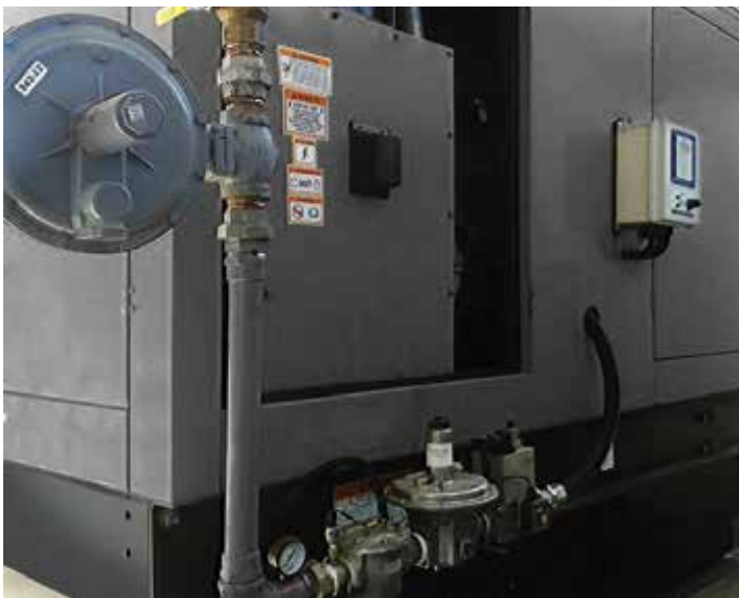
Peak Shaving/Standby (Propane)
