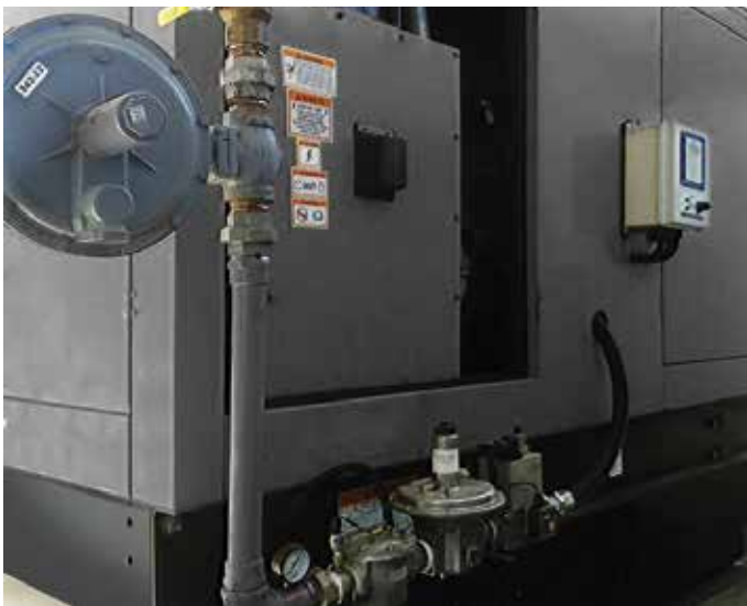
Peak Shaving/Standby (Propane)
